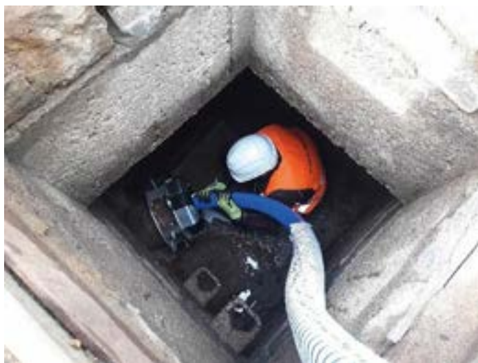
Existing manholes can be used as access points for trenchless rehabilitation
