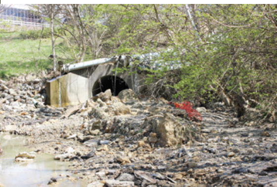
Debris Collecting at the Failed Culvert
