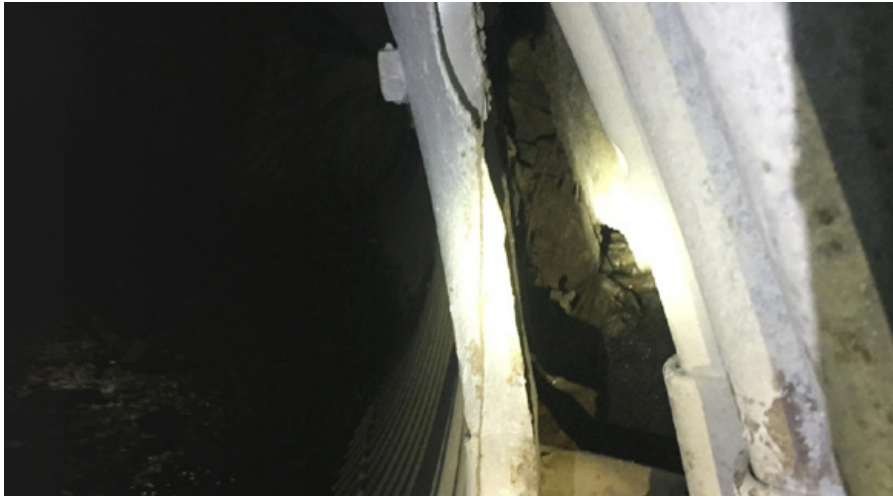
Multiple pipe joints were separated
