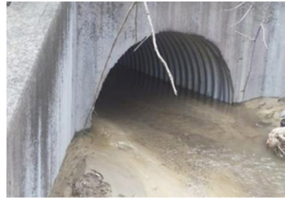
Due to accelerated corrosion, culvert had significantly deteriorated
