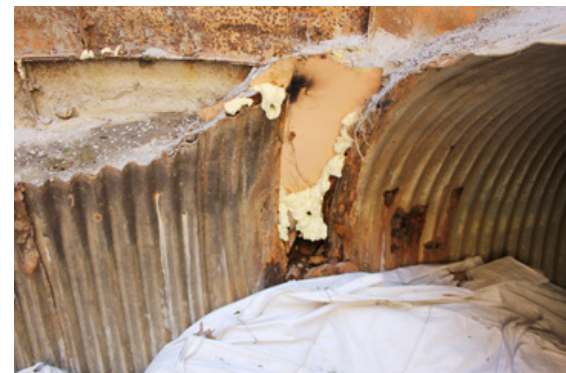
Failure showing welded joints coming apart
