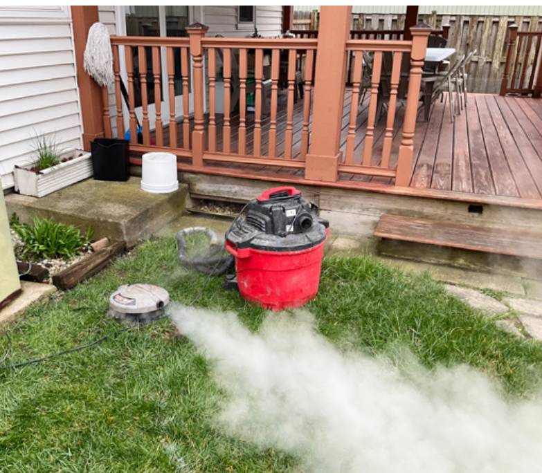
Figure 8. Steam Curing Process – upstream volatile organic compound relief at Vac-A-Tee
