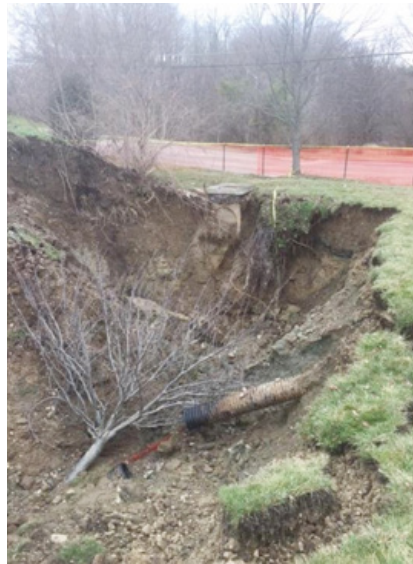
Massive sinkhole caused by failed culvert
