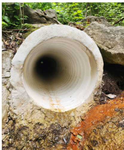
A structural, stand-alone pipe within the original sewer
