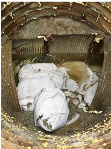
Debris found within culvert pipe
