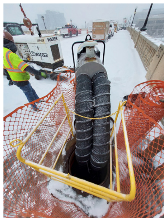
Blower heaters were installed in the access manholes on the bridge deck and within the access chambers beneath the bridge
