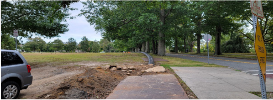
Figure 15: Buried by-pass piping at the Senior Center
