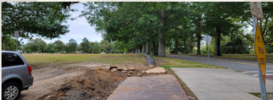
Figure 15: Buried by-pass piping at the Senior Center
