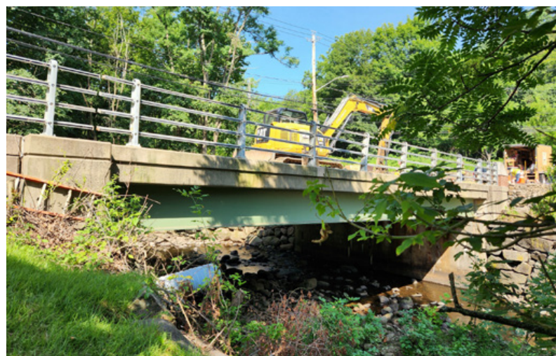
The 12-inch Ductile Iron water main runs under the Rosman Road bridge, spanning Minisceongo Creek
