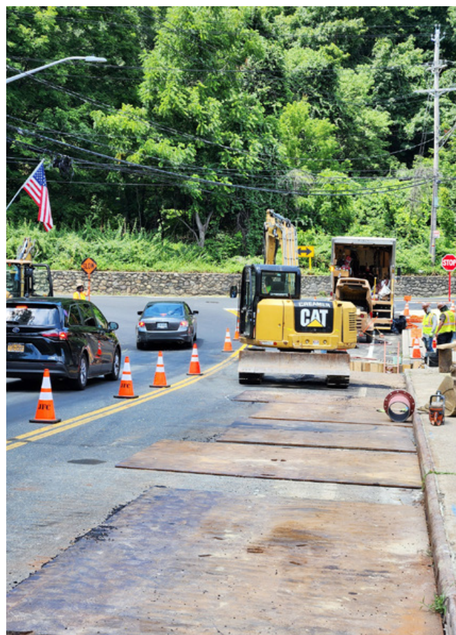
Watermain was fully restored to service within 48 hours
