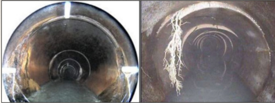
Figure 5: Typical defects observed along the GSC and broken pipe along the 18-inch diameter lateral sewer
