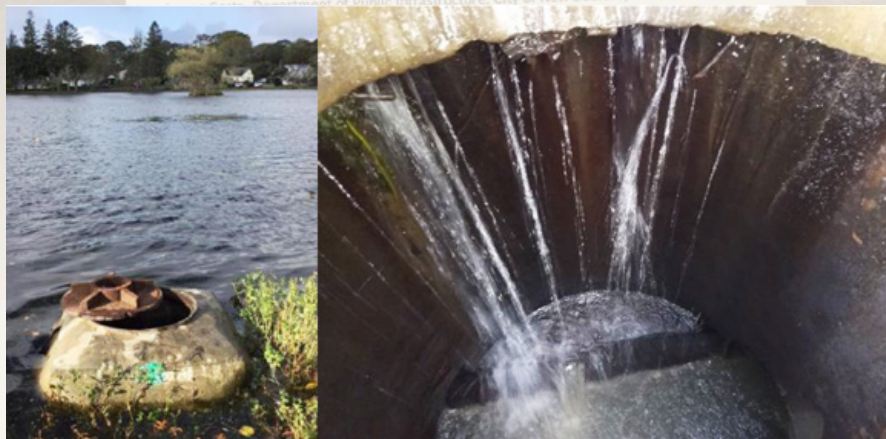
Figure 2: Manhole MH-5035 within Buttonwood Park Pond allowed inflow from the pond to enter the City's collection system.
