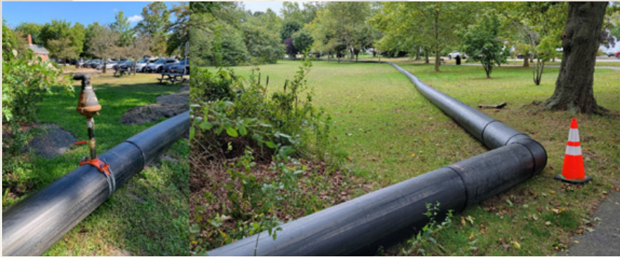
Figure 16: Typical Air Release Valve and Above Ground Piping
