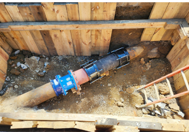
Repair clamp did not fully resolve the issue
