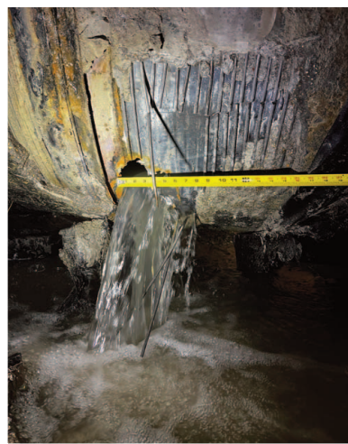
Figure 5. Leak that Occurred During the Condition Assessment
