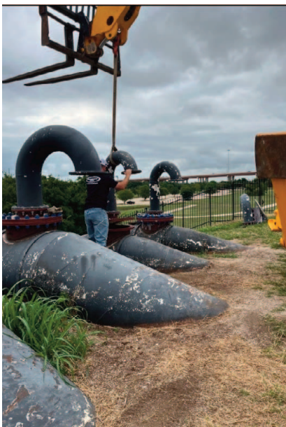
Figure 5. Vents with New Access Manways (Source: Stephens and Peterie 2025)
