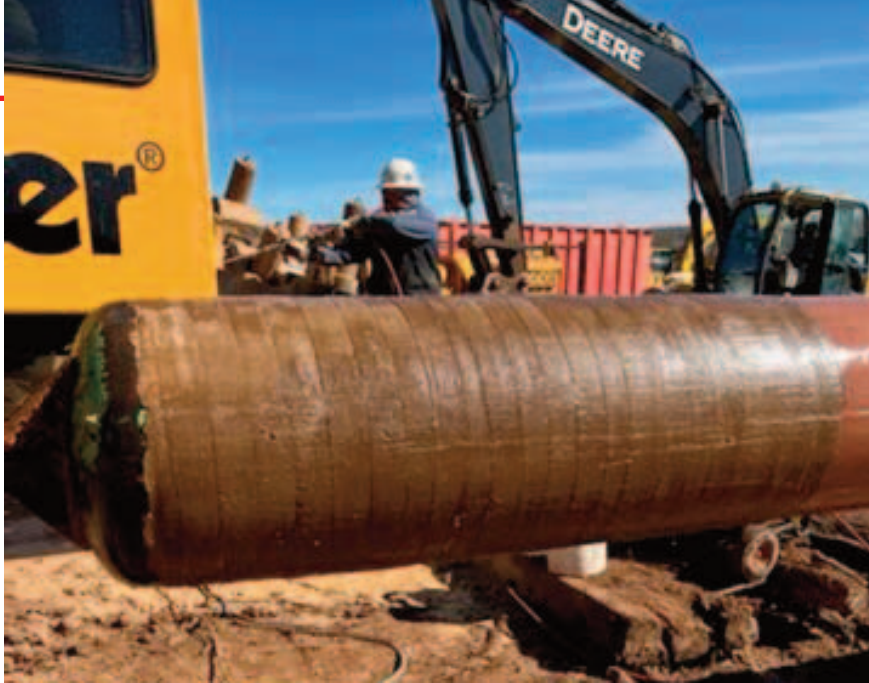
4-layer Bore-Wrap section showing only superficial scratches, with anti-corrosion layer fully preserved
