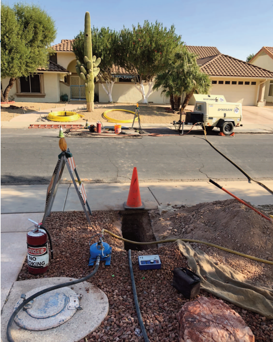
A typical piercing tool gas service installation jobsite layout. Note the minimal disruption of the trenchless application
