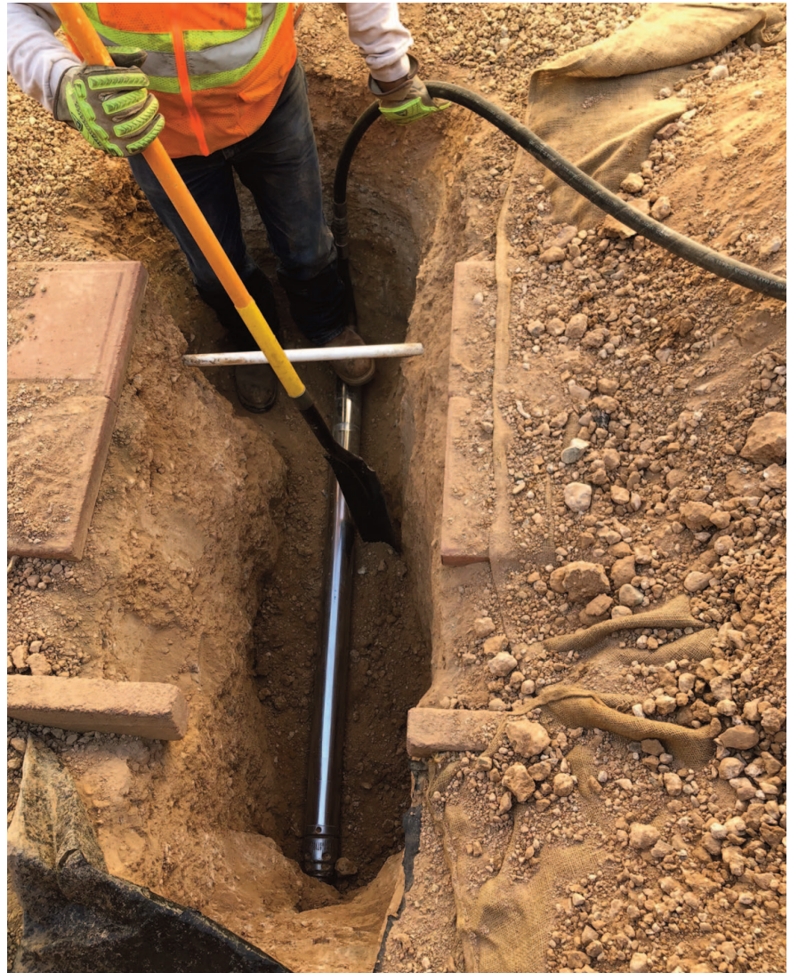
The piercing tool is a workhorse of the gas industry. Shown here, a Grundomat piercing tool is ready to go, in the launch pit, on a gas service installation project
