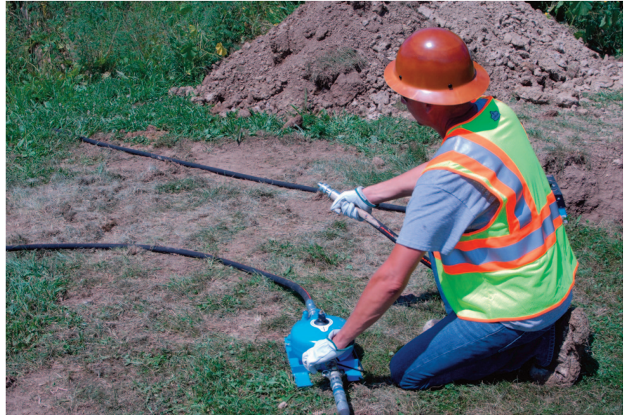
Ensuring proper lubrication during use is accomplished through an inline lubricator. Here, the operator checks lubricator operation before final piercing tool set up
