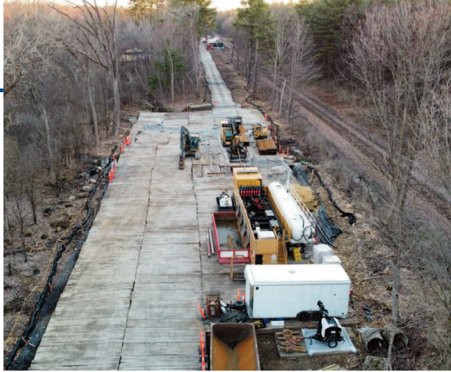
Longer bores, tighter tolerances and more complex pipe strings are becoming increasingly common
