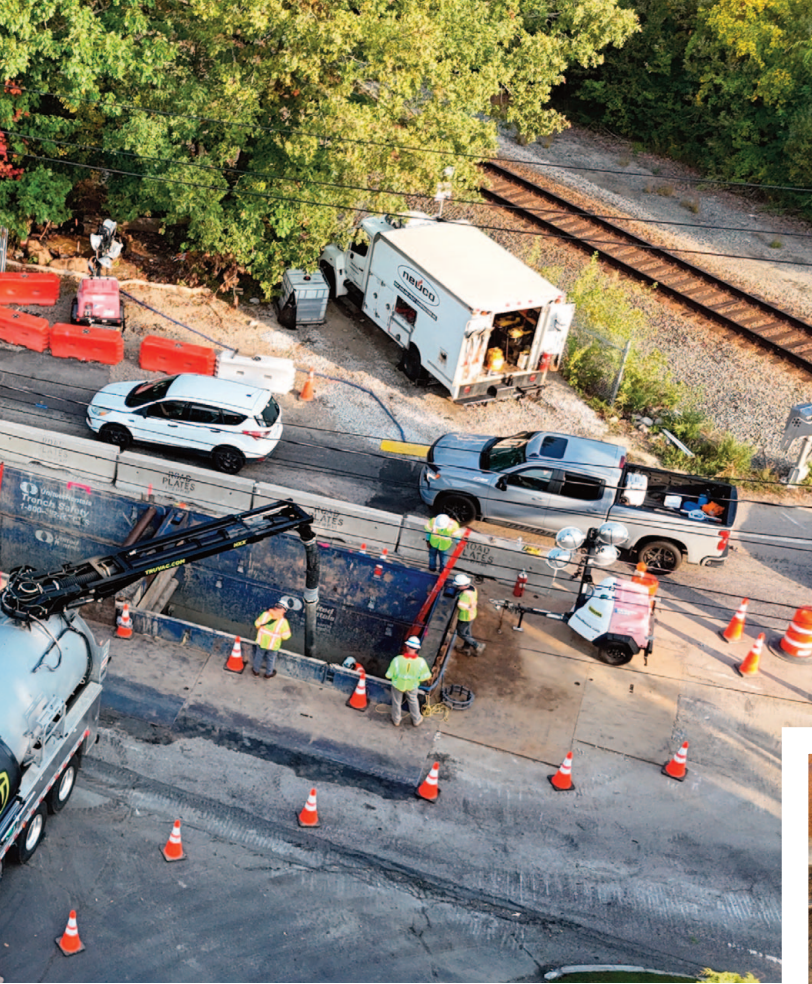
A new 12-inch gas main was installed below a high speed MBTA track.
