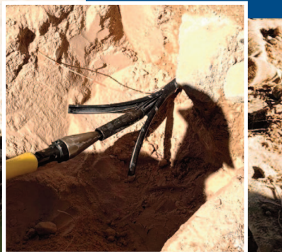
Trenchless split and pull replacement is paired with minimally invasive excavation and restoration techniques
