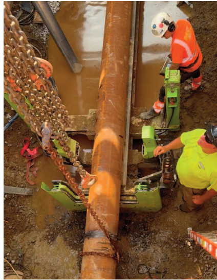
Chains were used to rotate the casing in order to finish welding the sections
