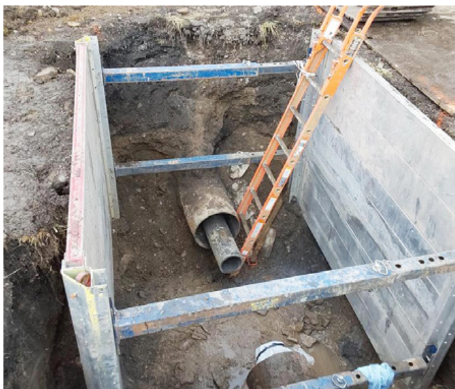
Cast iron water main was found to be encased within a 16 inch steel casing
