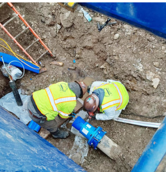
Primus Line® rehabilitation system was determined to be the most effective long-term solution
