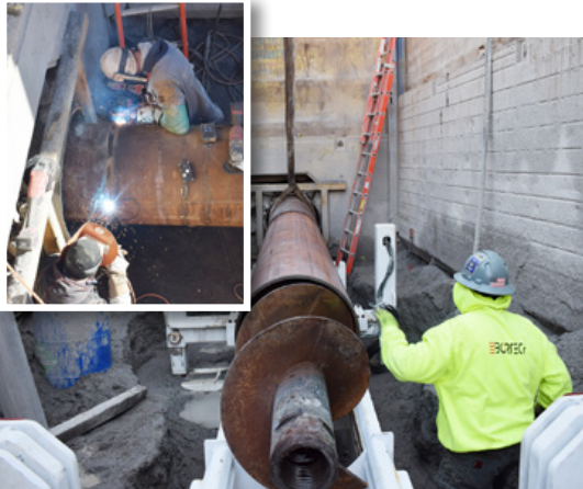
A project-specific centralizing system guided the 24-inch casing through the predrilled alignment while maintaining strict line and grade tolerances
