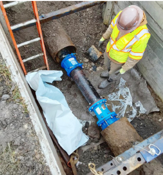
Available records on the pipeline installation were extremely limited
