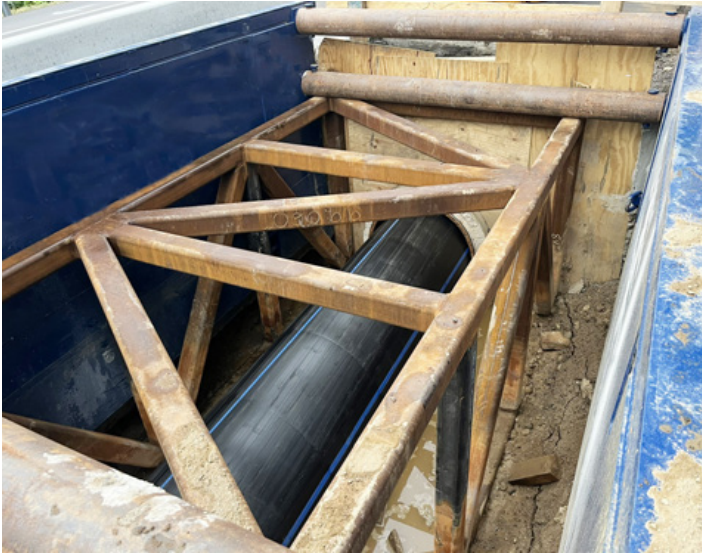
The 42-inch-diameter PE4710 HDPE is fed through the Murphy Pipeline compression die into the old 42-inch prestressed concrete cylinder pipe (PCCP)
