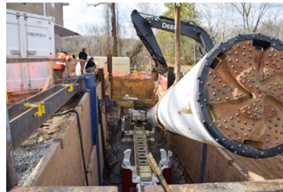
The 36-inch starter casing was precision-positioned to establish initial line and grade control for the telescoping installation
