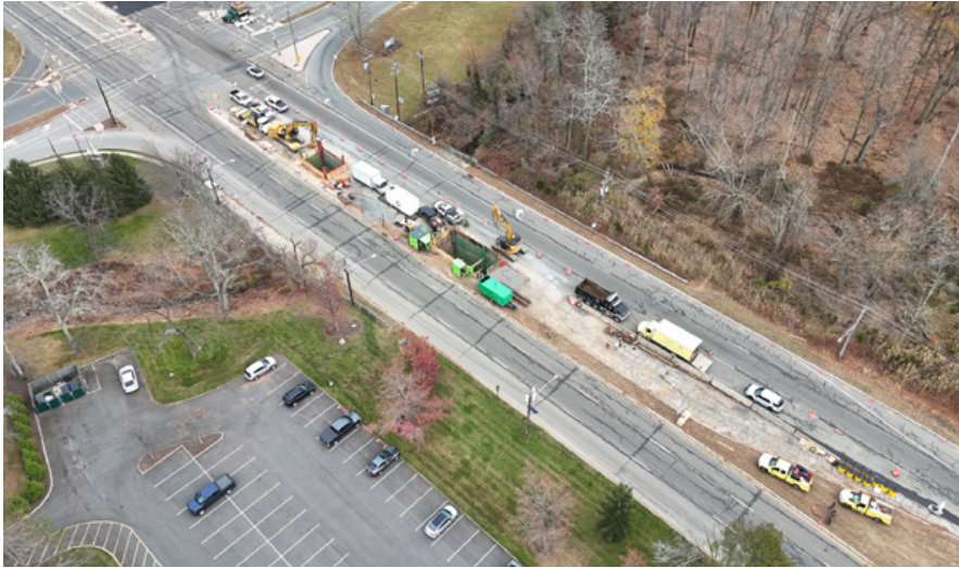
Several projects in the Northeast have been specifically designed to utilize the HHB method
