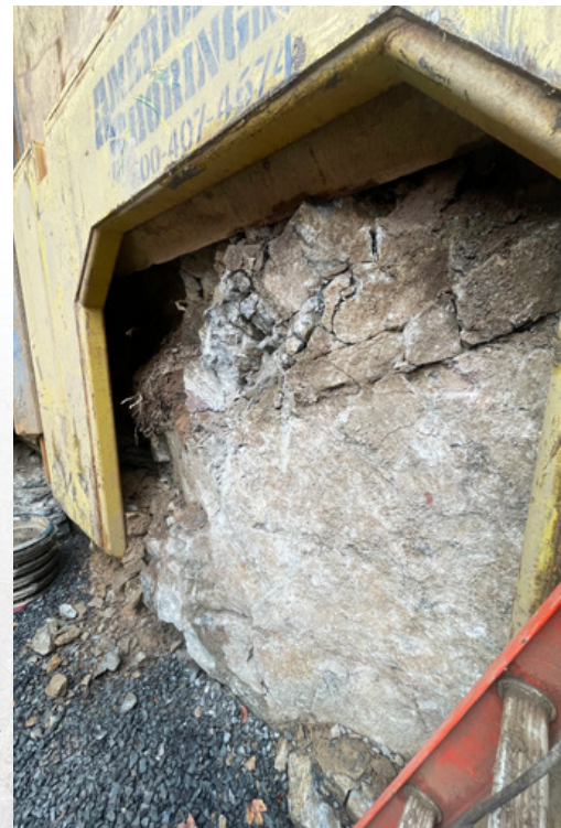
Subsurface conditions consisted of highly competent granitic gneiss with elevated abrasivity throughout the alignment
