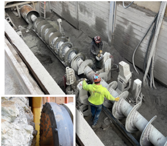
Removal of the downhole hammer assembly following completion of the initial 36-inch telescoping phase
