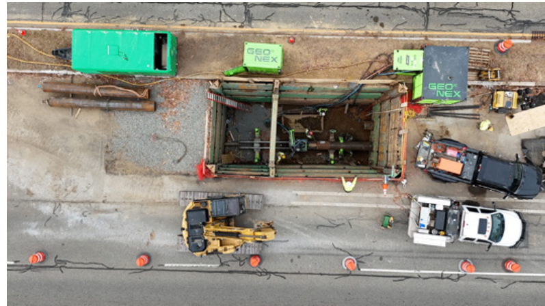
Figure 5. Aerial view of HHB System deployed in a highway median
