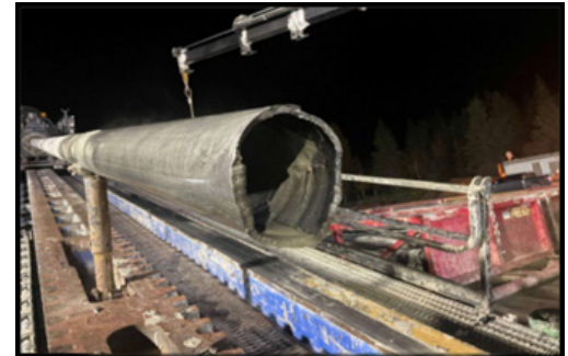
Figure 11 - Drill Pipe String break #1
