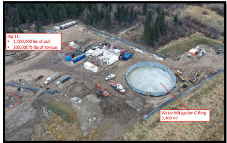
Figure 9 – Additional containment for Drilling Fluid
