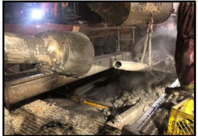
Figure 13 – Drill Pipe break #1
